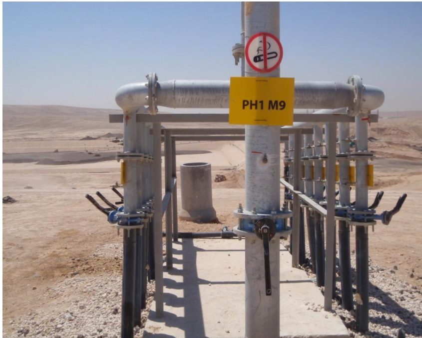
Manifold with gas pipe connection and numbers
